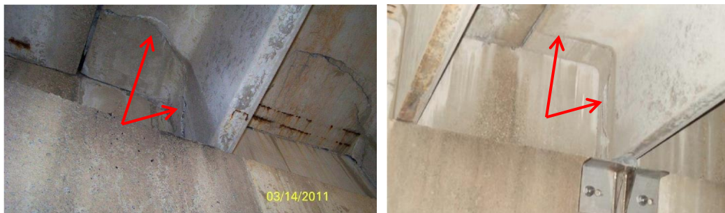
Figure 1. Crack observed in Double Tee Canopy Beam(Haraway, 2015)
