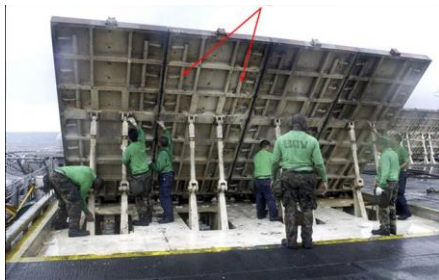
Figure 2. Jet blast deflector being serviced aboard a Navy ship.
