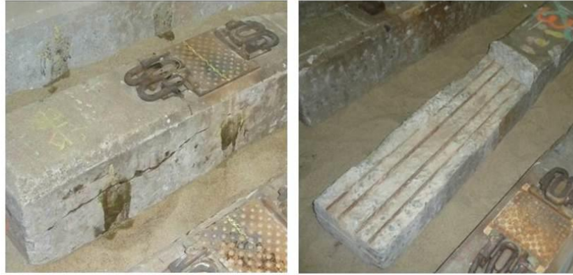
Figure 1. Example pictures of concrete cross-ties with horizontal cracks (Mayville et al. , 2014).
