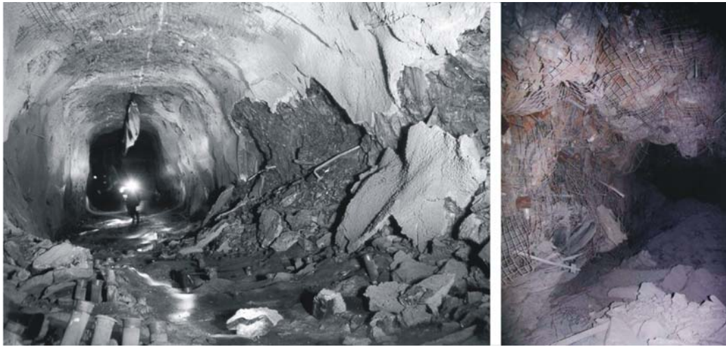
Figure 1. Examples of Moderate to Significant Damage (Photograph by Capes, 1999, left) and Significant to Very Significant Damage (right)
